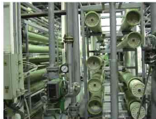
Low-pressure Filtration System
