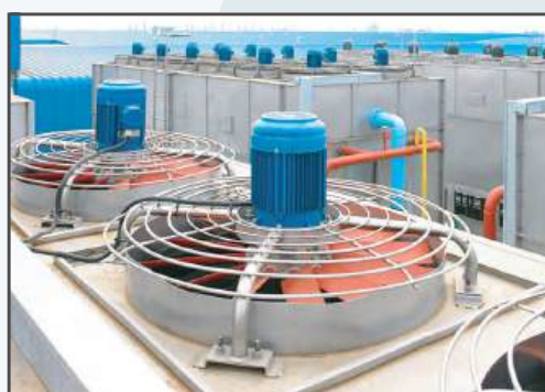
Fan and water pump
