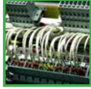
Electrical cabinets and substations
