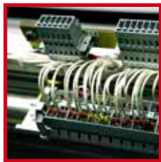
Electrical cabinets and substations
