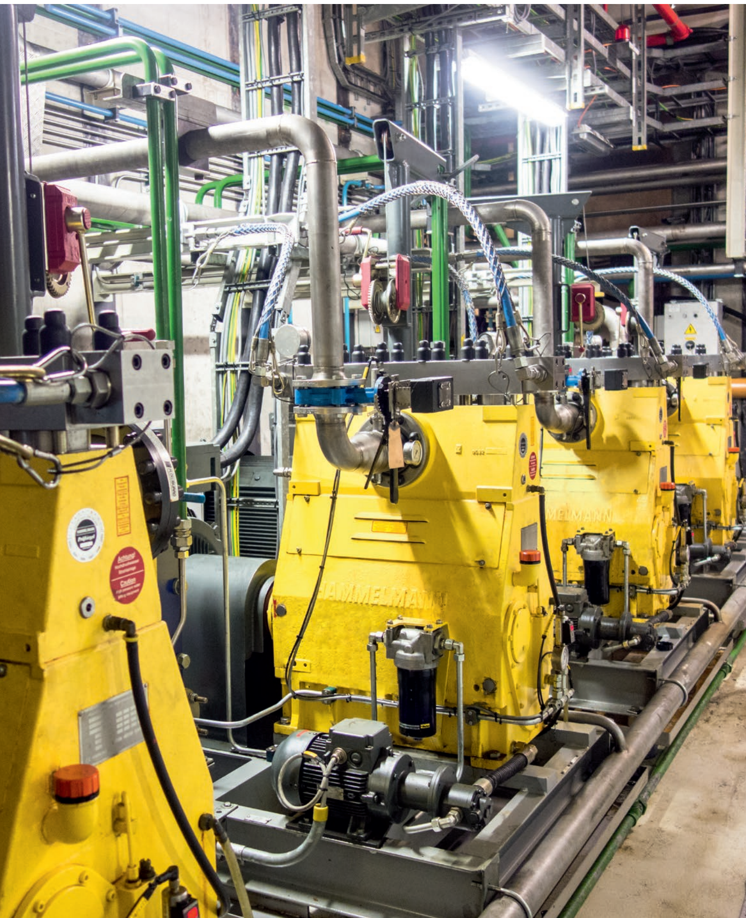
High pressure pumps in the aluminium industry. Above in operation since 2009 with an average of 5000 operating hours per year.
