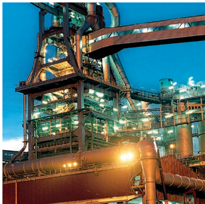
Industrial application: Refinery
