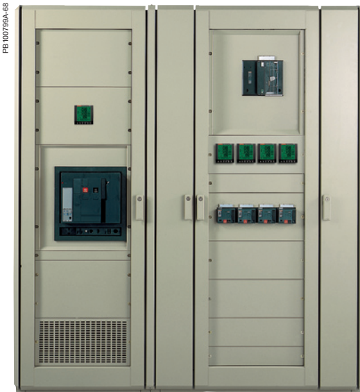
Main LV switchboard.
